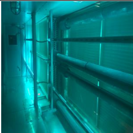
AHU Cooling Coil
