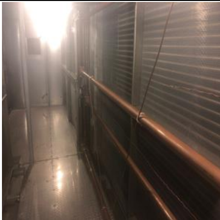
AHU Heating Coil
