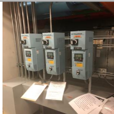
AHU Electrical connections
