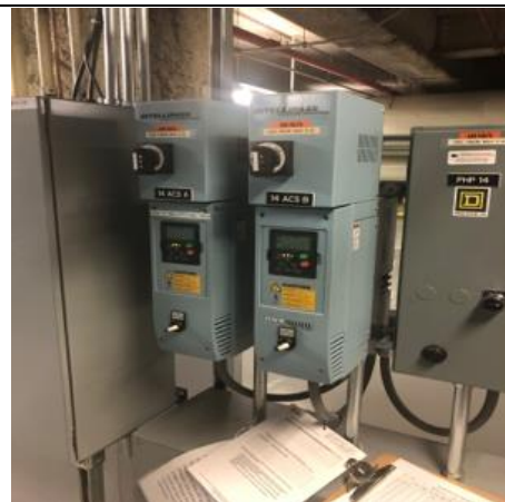
AHU Electrical connections
