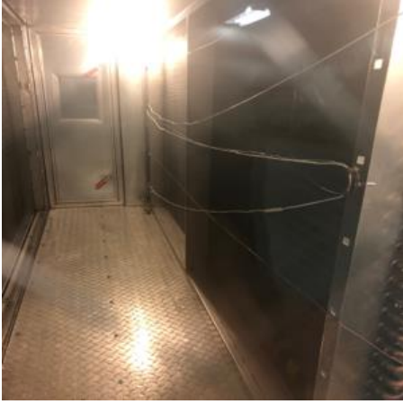
AHU Heating Coil
