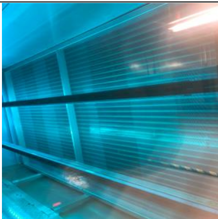
AHU Cooling Coil
