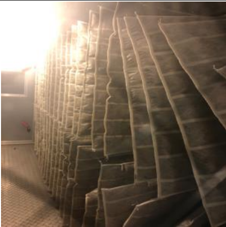
AHU Final Filter
