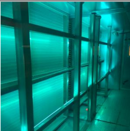
AHU Cooling Coil
