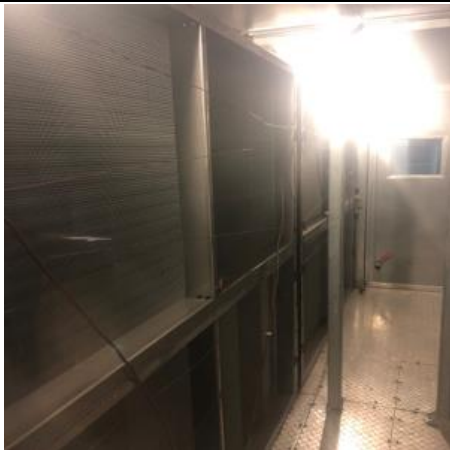
AHU Heating Coil
