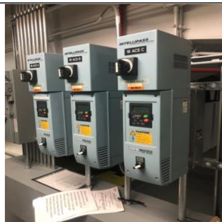
AHU Electrical connections
