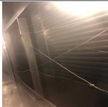
AHU Heating Coil
