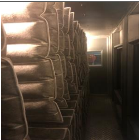
AHU Final Filters
