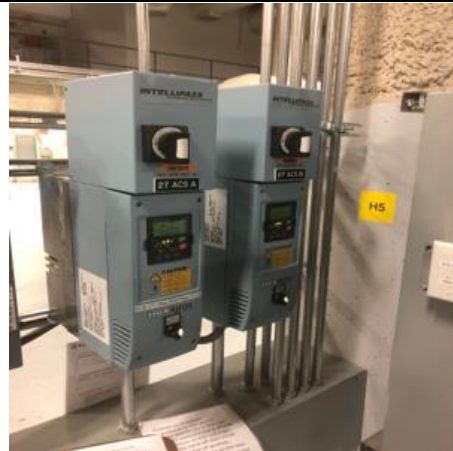
AHU Electrical connections
