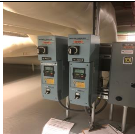
AHU Electrical connections
