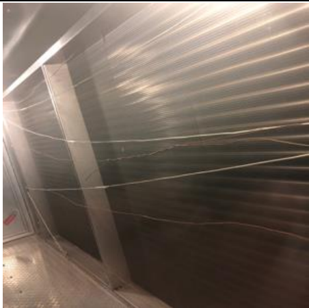
AHU Heating Coil
