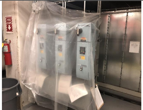
AHU Electrical Connections
