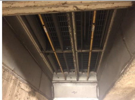
AHU OA Intake 2
