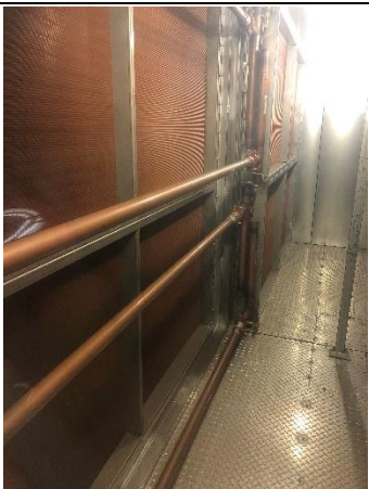
AHU Heating Coil
