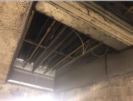
AHU OA Intake 1
