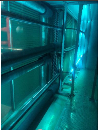
AHU Cooling Coil
