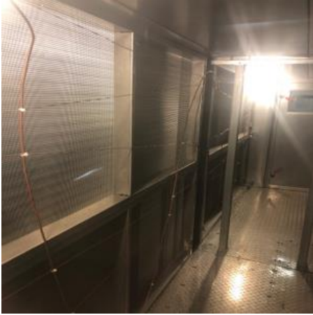
AHU Heating Coil
