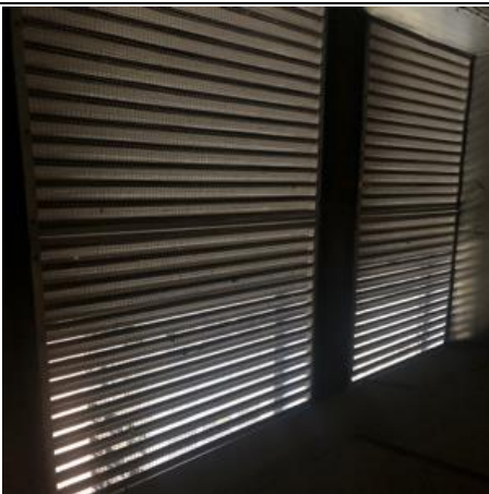
Outdoor Air Intake
