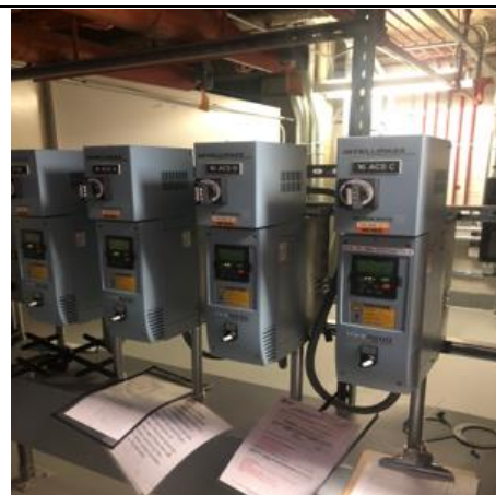
AHU Electrical connections
