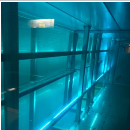
AHU Cooling Coil
