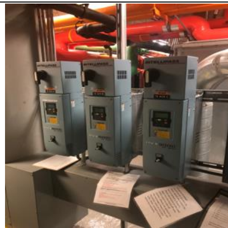
AHU Electrical connections
