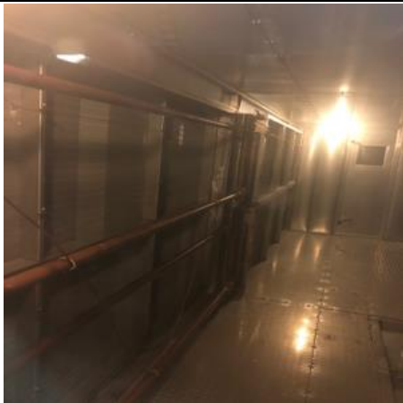
AHU Heating Coil
