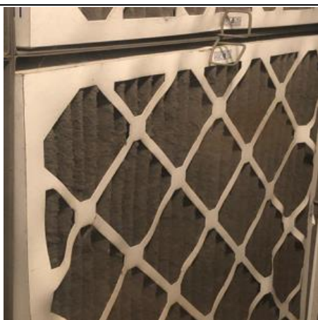
Dirty Filters Observed
