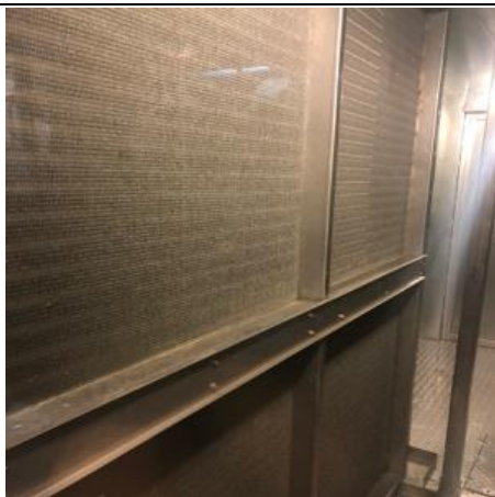
AHU Heating Coil
