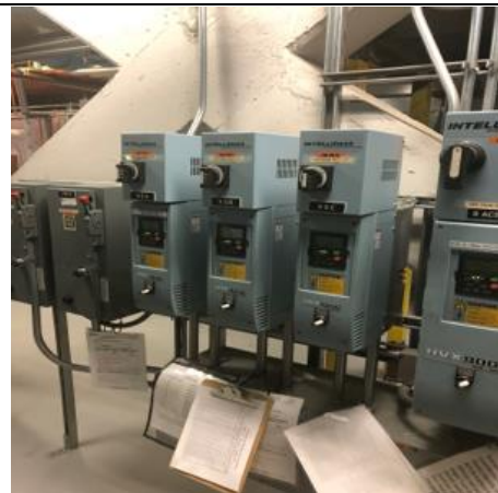
AHU Electrical connections
