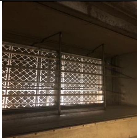
AHU OA Intake
