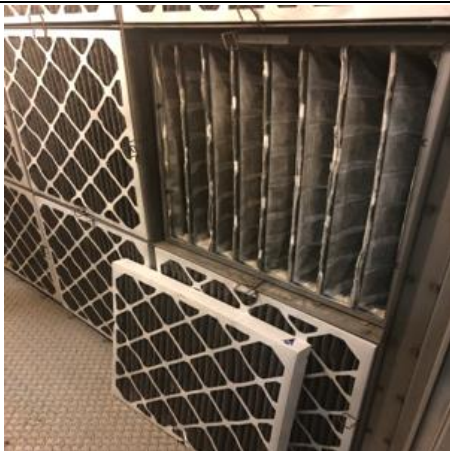
AHU Filters Recommend Replacing
