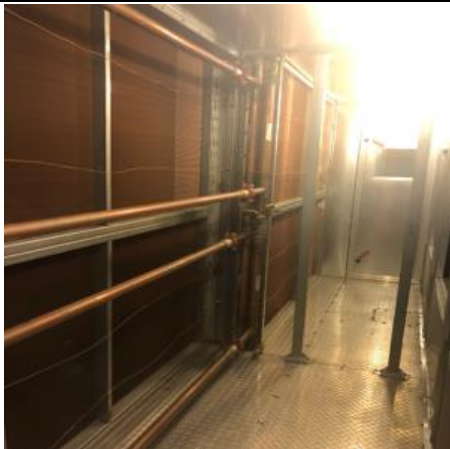
AHU Heating Coil
