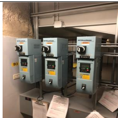
AHU Electrical connections
