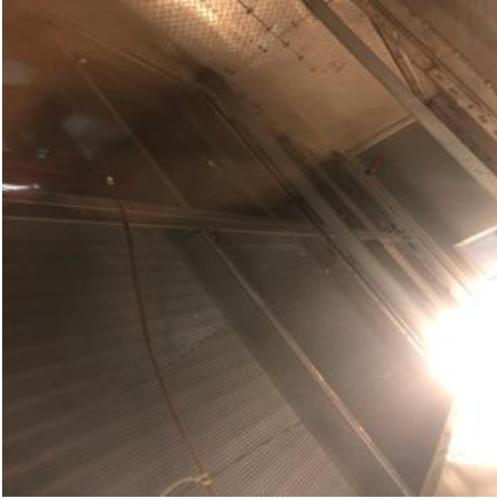
AHU Heating Coil
