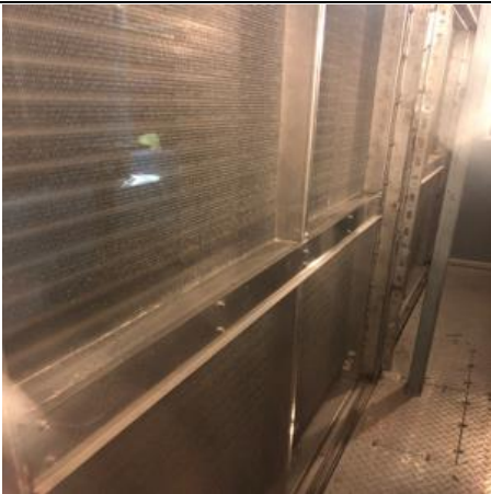
Dusty Heating Coil observed
