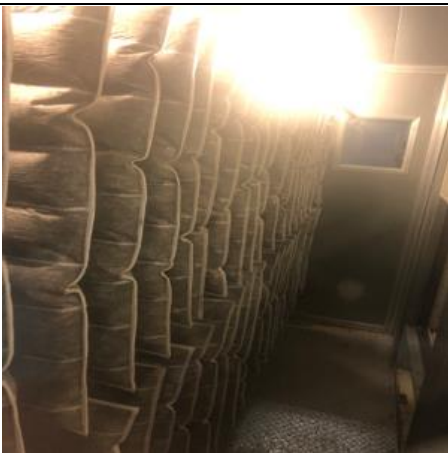
AHU Final Filter
