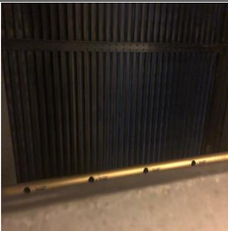
Outdoor Air Intake
