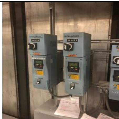
AHU Electrical connections
