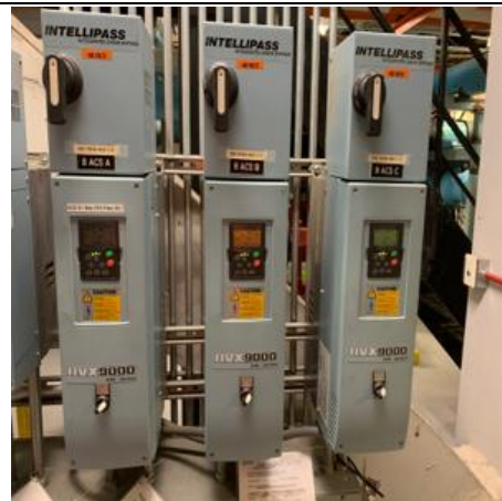
AHU Electrical connections
