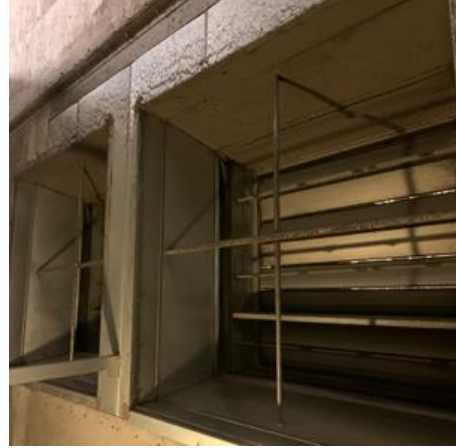
AHU OA Intake
