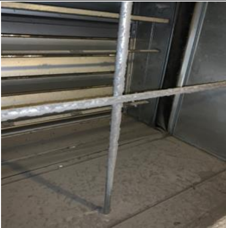
AHU OA Intake
