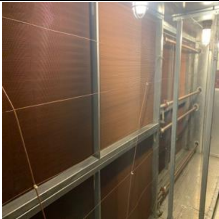
AHU Heating Coil
