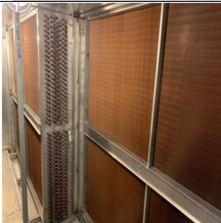
AHU Cooling Coil
