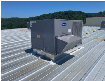
RTU3 Unit picture
