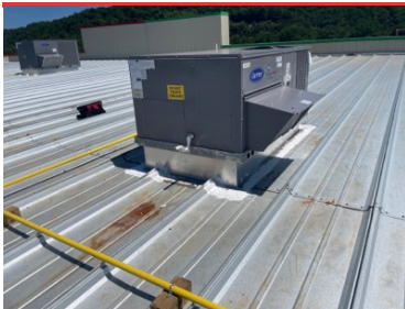
RTU1 Unit picture
