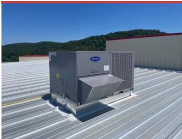
RTU2 Unit picture
