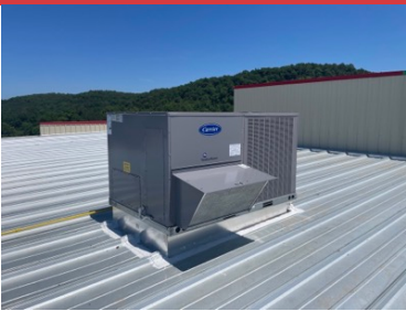
RTU2 Unit picture
