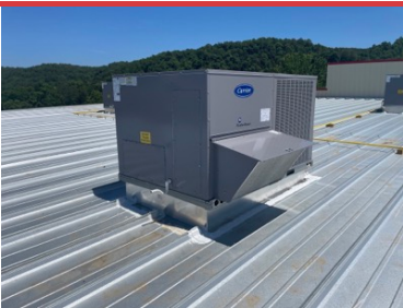
RTU3 Unit picture
