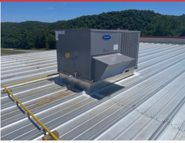
RTU4 Unit picture
