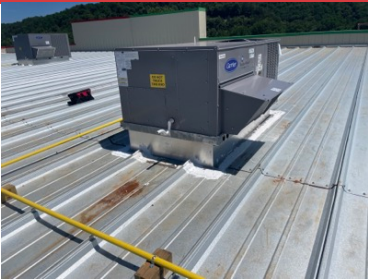
RTU1 Unit picture
