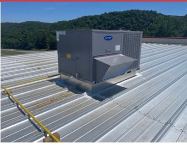
RTU4 Unit picture
