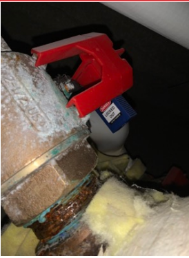
CHILLED WATER VALVES LOCKED OUT
