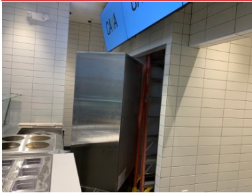
ACCES TO AHUS/ BALANCE VALVES
