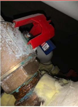
CHILLED WATER VALVES LOCKED OUT
