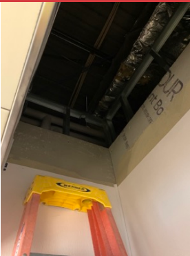
ACCESS TO AHUS AMD BALANCE VALVES
