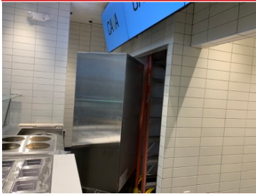
ACCES TO AHUS/ BALANCE VALVES
