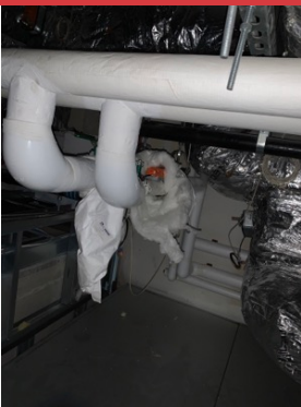
AHU-2 BALANCE VALVE
