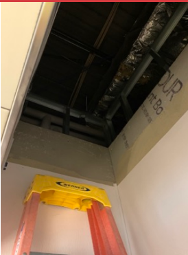
ACCESS TO AHUS AMD BALANCE VALVES
