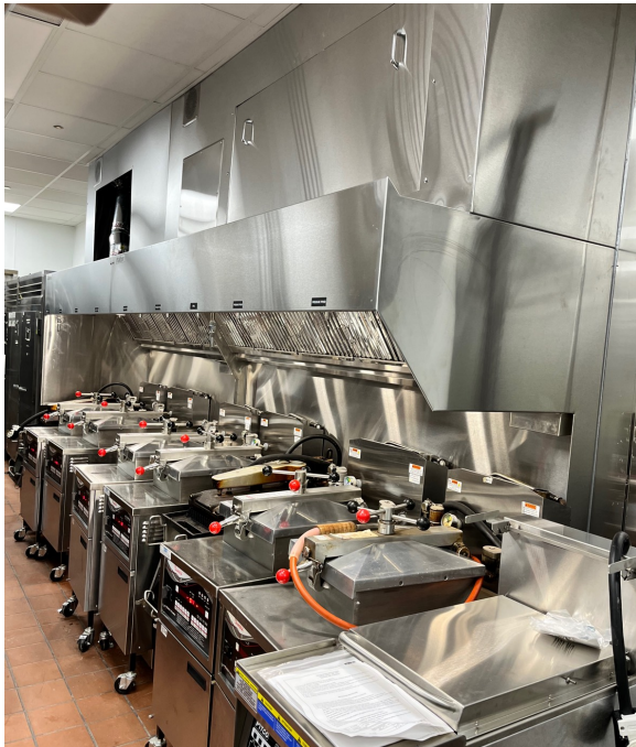
Deep Fryer Hood
