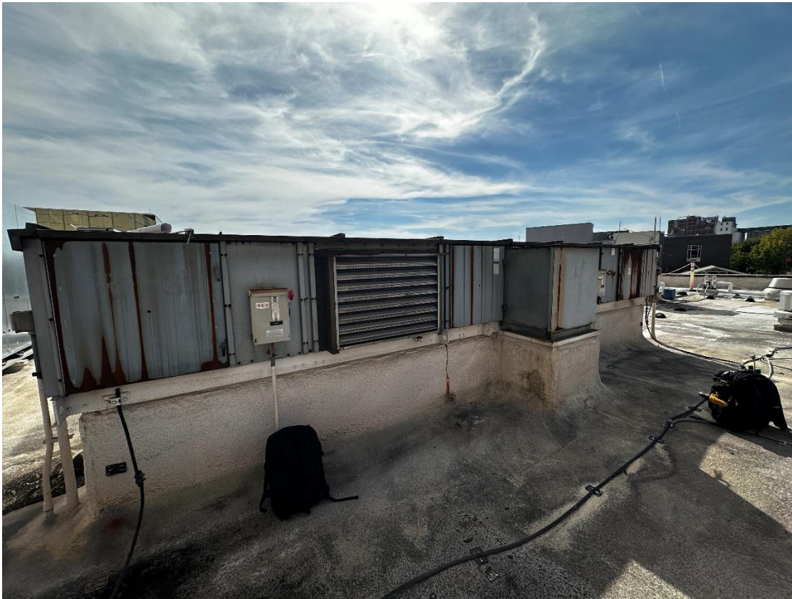
AHU-31 located up on Roof
