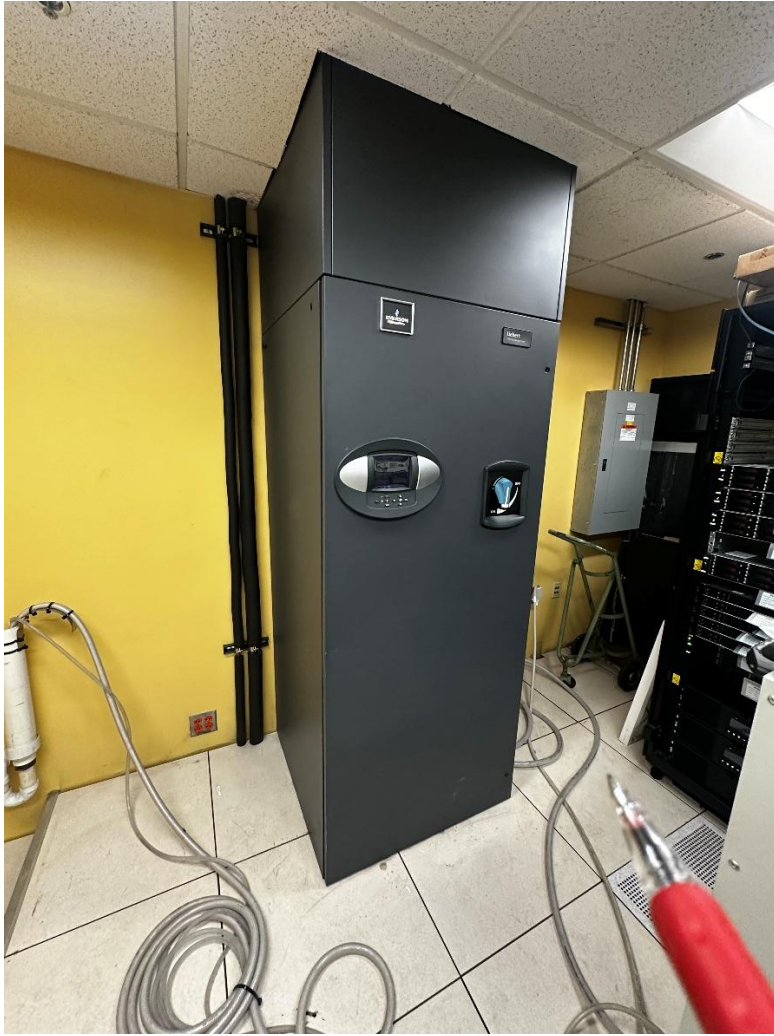
New data room with Liebert unit next to room B-3034
