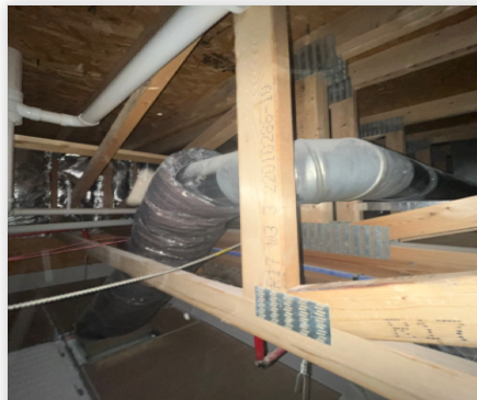
Ductwork above restroom.. 07/19/2023
