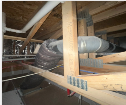
Ductwork above restroom.. 07/19/2023
