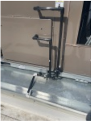
Installed RTU Condensate Drain Photo
