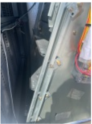
Completed RTU Economizer Damper Linkage Photo
