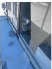
Installed RTU Gas Heat Vent Hood Photo
