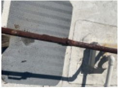
RTU Gas Shut-Off Valve in ON Position Photo
