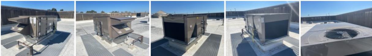
All 5 Sides of Installed Unit of RTU - Including Top with Condensor Fan Section.
