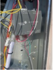
Installed RTU Economizer Photo
