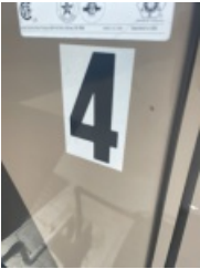
RTU Label Photo
