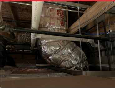
HD-1 GREASE DUCT
