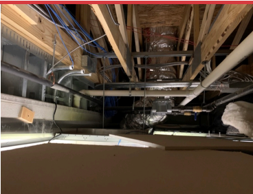
HD-2 GREASE DUCT
