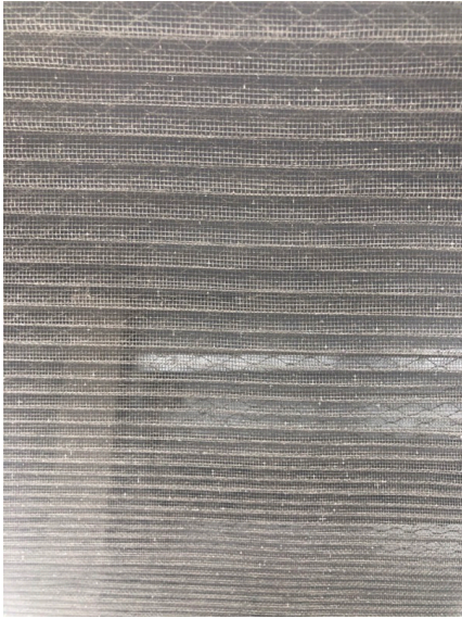
RTU-1 Dirty outside air filters
