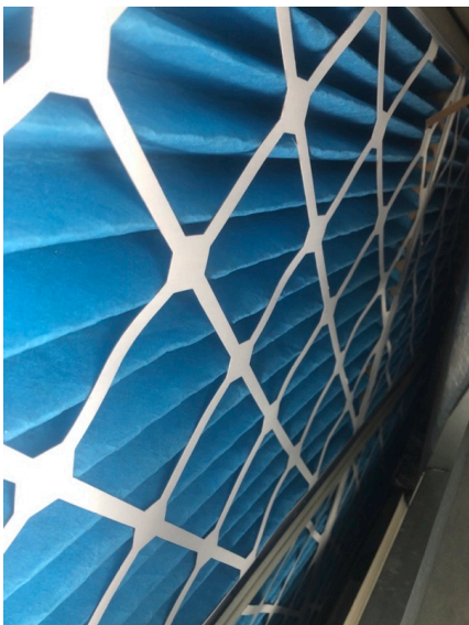
RTU-1 Clean evaporator filters
