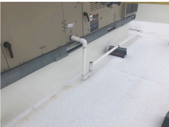
RTU-2 Condensate drain
