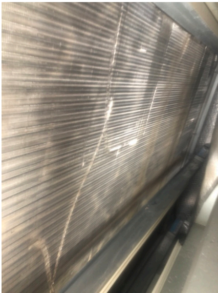
RTU-2 Dirty evaporator coil
