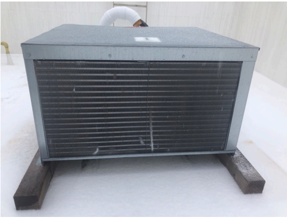
Walk-in Freezer Dirty condenser
