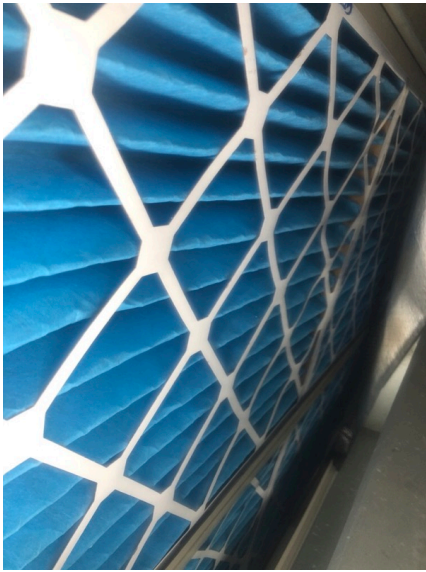
RTU-2 Clean evaporator filters
