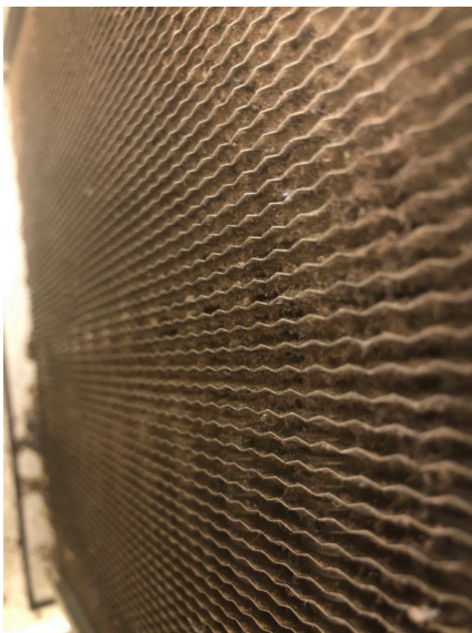
Fryer Freezer Clean condenser
