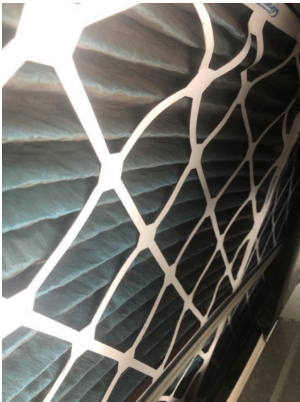
RTU-1 Dirty evaporator filters
