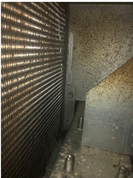
Meat Cooler 1 Clean condenser
