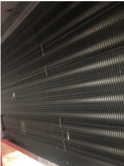
Walk-in Freezer Dirty evaporator
