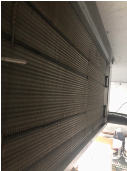
Walk-in Cooler Dirty evaporator
