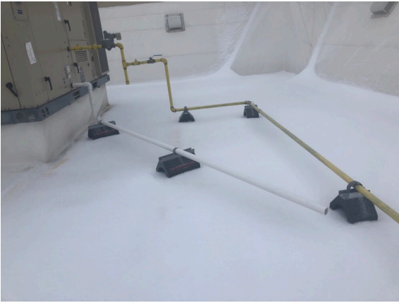
RTU-1 Condensate drain
