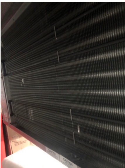
Walk-in Freezer Clean evaporator
