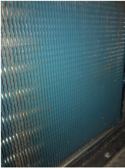
Toppings Clean condenser
