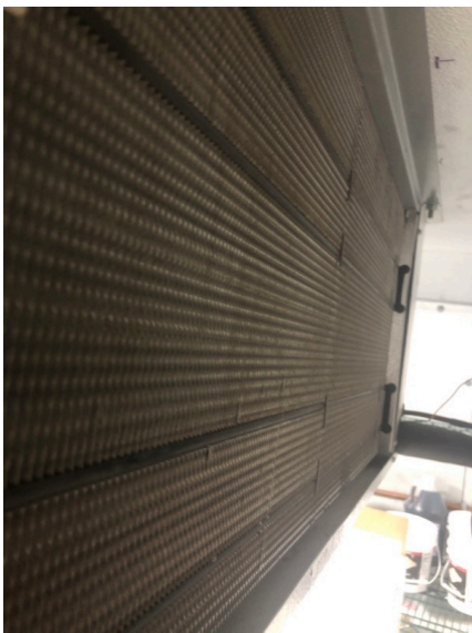
Walk-in Cooler Clean evaporator
