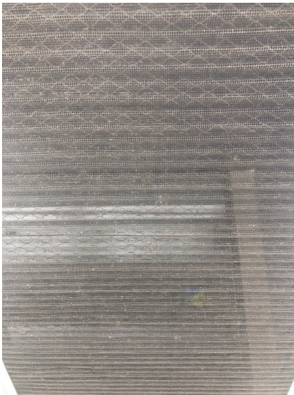
RTU-2 Dirty outside air filters
