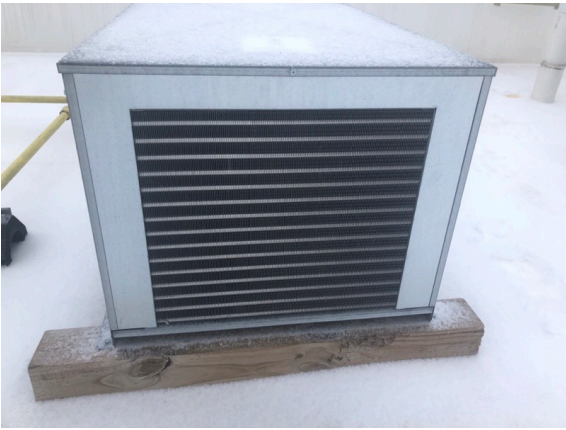
Walk-in Cooler Dirty condenser
