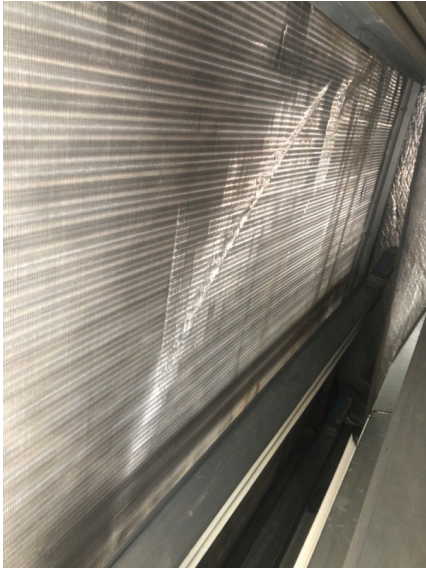
RTU-1 Dirty evaporator coil
