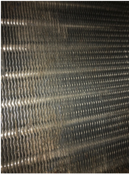
Prep Table 1 Clean condenser
