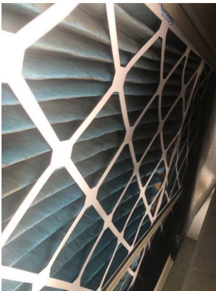
RTU-2 Dirty evaporator filters
