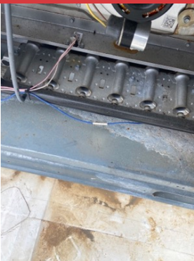
RTU-2 HEATING COMPARTMENT
