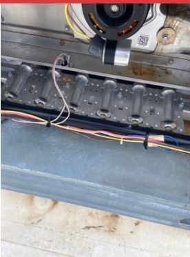
RTU-2 HEATING COMPARTMENT
