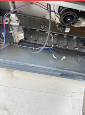
RTU-1 HEATING COMPARTMENT
