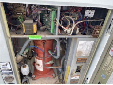
OFFICE RTU4 ELECTRICAL COMPARTMENT
