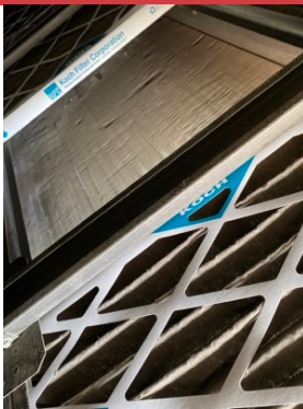
RTU SOUTH EVAPORATOR COIL
