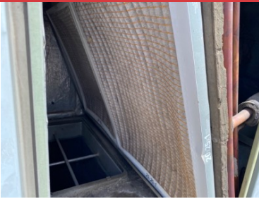
PHARMACY RTU3 FILTERS
