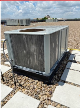
PHARMACY RTU3 CONDENSER COIL
