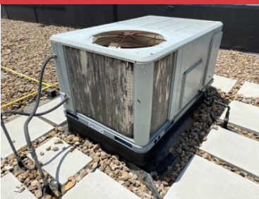
BAKERY RTU5 CONDENSER COIL Damaged fins
