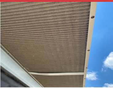
RTU5 BAKERY O/A FILTER Dirty
