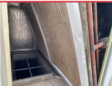
OFFICE RTU4 FILTERS
