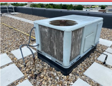
OFFICES RTU4 CONDENSER COIL
