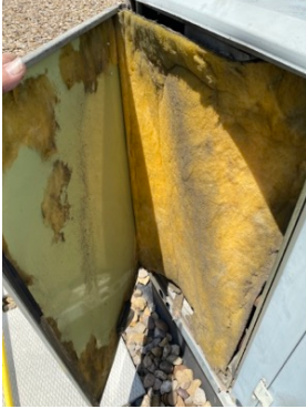
BAKERY RTU5 LOOSE INSULATION
