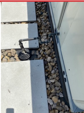
BAKERY RTU5 DRAIN
