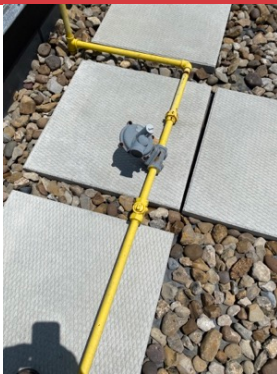
BAKERY RTU5 GAS VALVE
