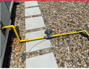
RTU NORTH GAS VALVE POSITION
