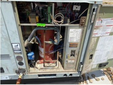
PHARMACY RTU3 ELECTRIC COMPARTMENT
