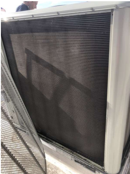
RTU-2 Clean condenser coil
