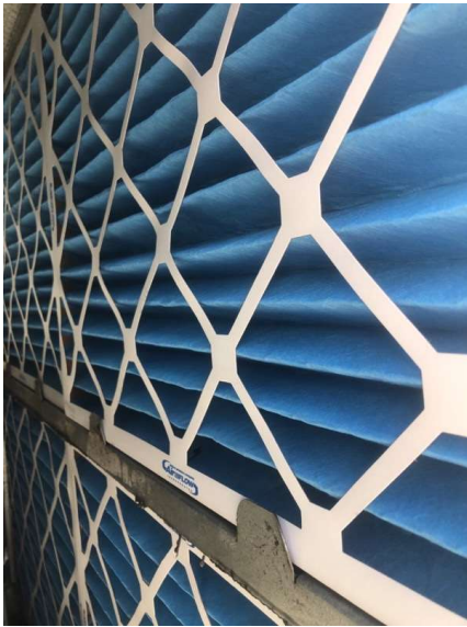
RTU-2 Clean evaporator filters
