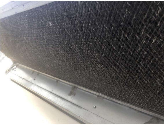
RTU-3 Dirty outside air filters
