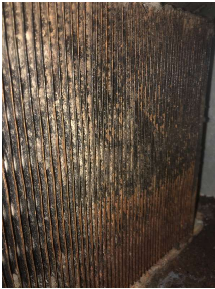
Toppings Clean condenser
