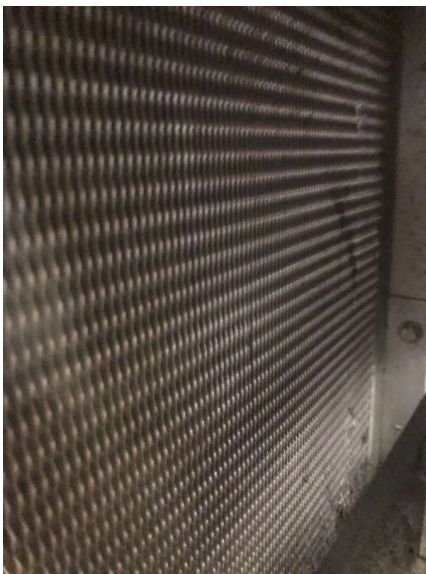
Meat Cooler 1 Clean condenser
