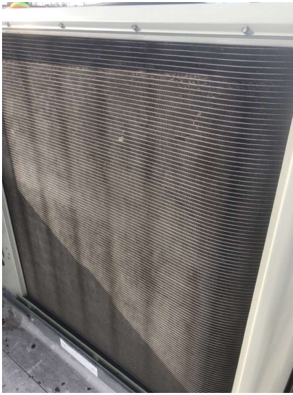
RTU-1 Dirty condenser
