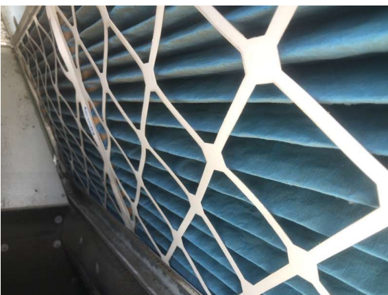
RTU-1 Dirty evaporator filters
