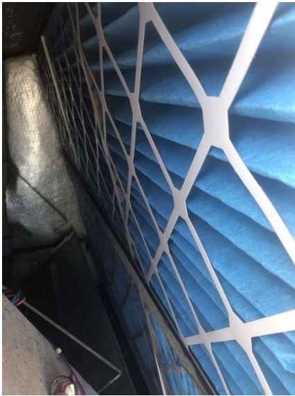
RTU-3 Clean evaporator filters
