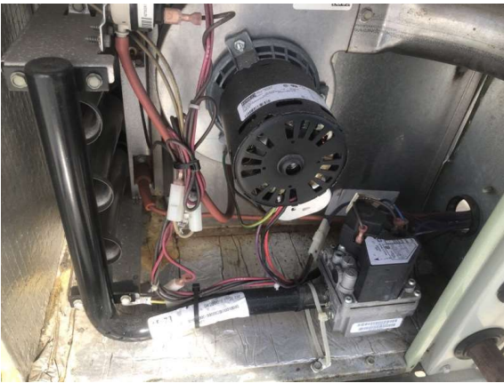
RTU-2 Heating compartment
