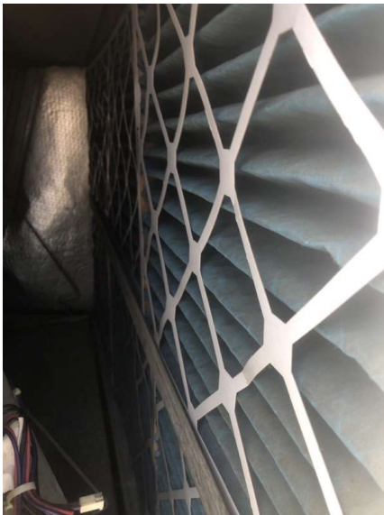
RTU-3 Dirty evaporator filters
