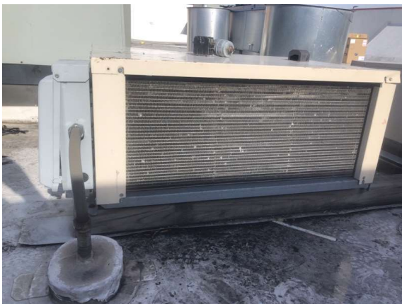
Walk-in Freezer Dirty condenser
