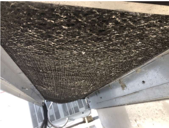
RTU-3 Clean outside air filters
