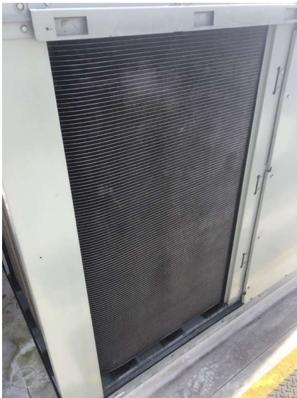
RTU-3 Clean condenser coil
