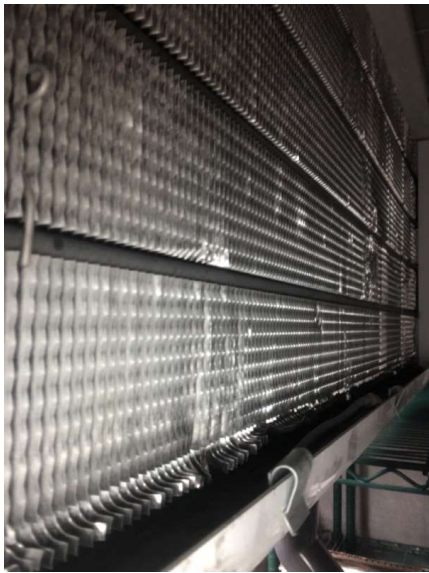
Walk-in Freezer Clean evaporator
