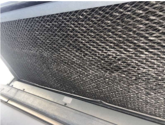
RTU-1 Dirty outside air filters
