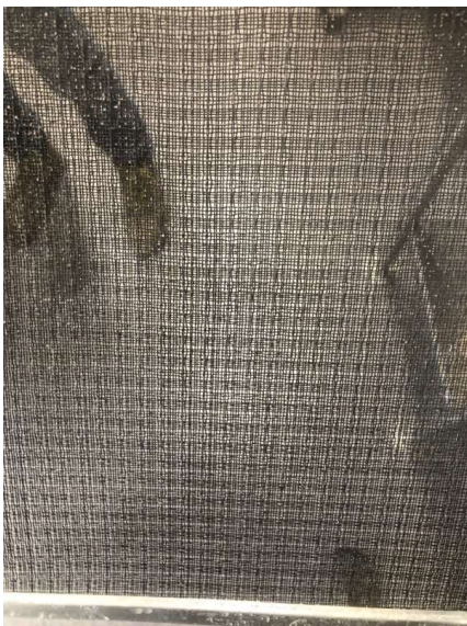
Fryer Freezer Clean condenser
