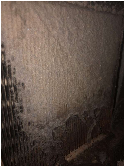
Toppings Dirty condenser
