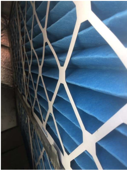
RTU-1 Clean evaporator filters
