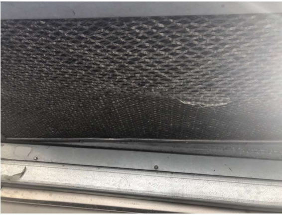
RTU-2 Dirty outside air filters
