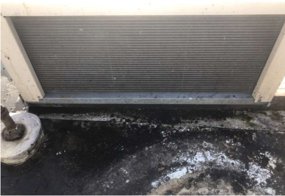
Walk-in Cooler Dirty condenser
