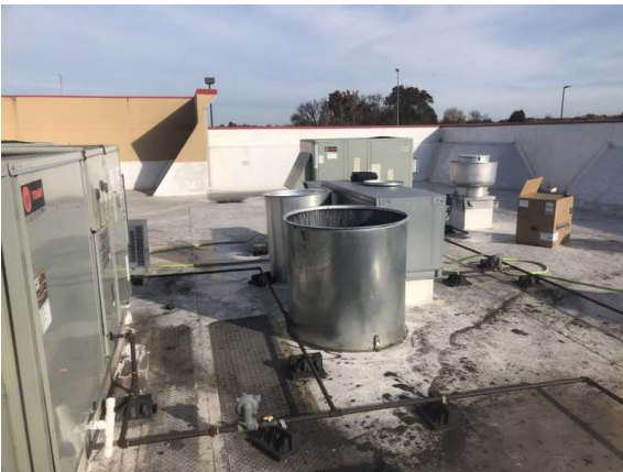
ISSUE: Wind Band Extensions Wind band extensions found off of fans. NTAB placed back on fans.
