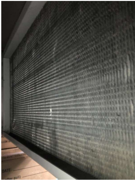
Walk-in Cooler Clean evaporator
