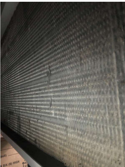
Walk-in Cooler Dirty evaporator
