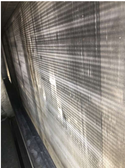
RTU-3 Dirty evaporator coil
