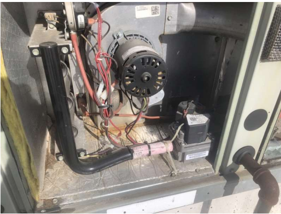
RTU-1 Heating compartment cleaned
