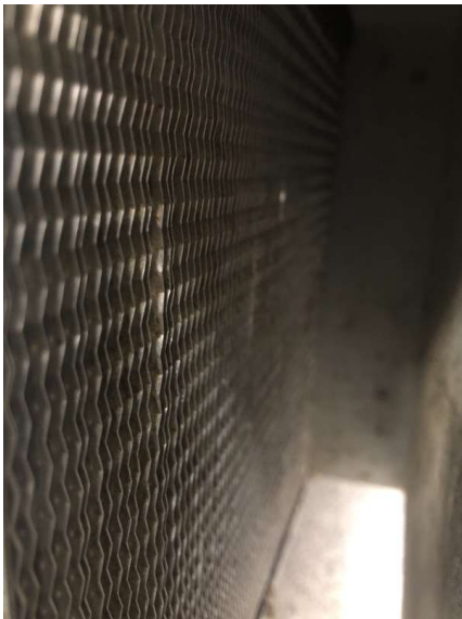
Meat Cooler 2 Clean condenser
