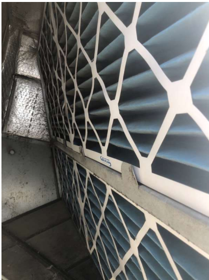
RTU-2 Dirty evaporator filters
