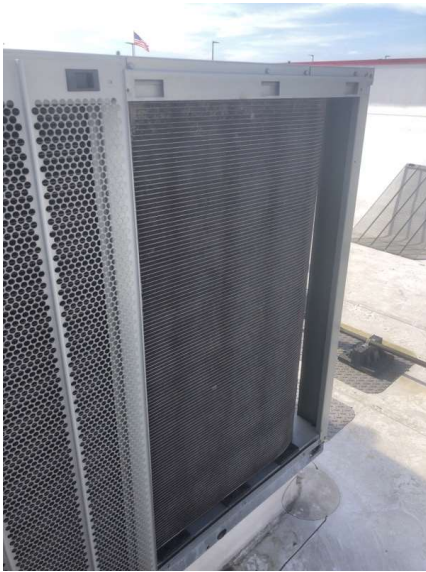
RTU-3 Dirty condenser coil
