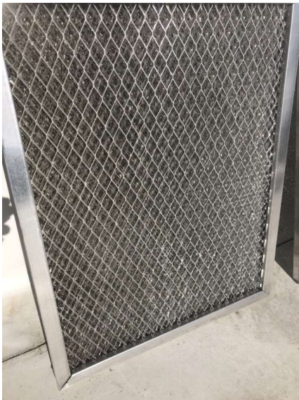
MAU Clean outside air filters
