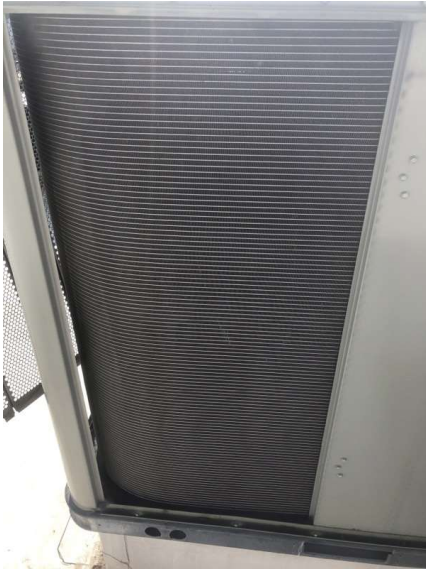
RTU-2 Dirt condenser coil
