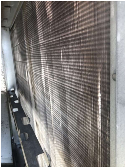
RTU-2 Dirty evaporator coil
