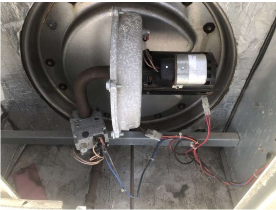
RTU-3 Heating compartment
