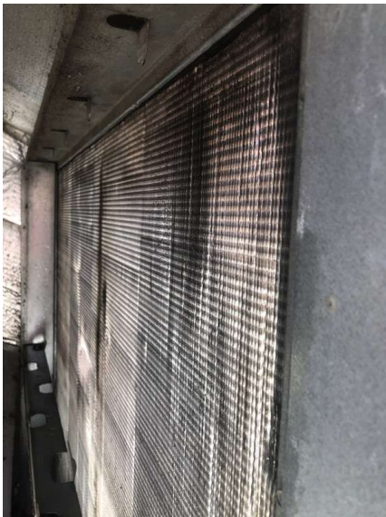
RTU-1 Dirty evaporator coil
