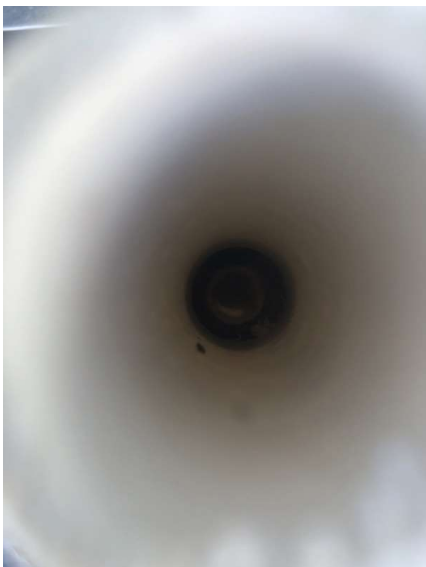
RTU-2 Condensate drain flushed clean
