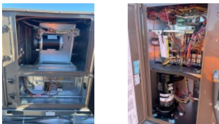
Interior Pictures of RTU Blower Section, Power / Control Section, Heat Section, Compressor Section.
