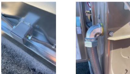
All RTU Electric and Heat Utility Piping Through Roof and All Connections / Penetrations at the Unit.
