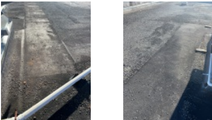
Roof Areas Around RTU Unit Showing the Areas are Clean and Free of Any Debris or Damage Related to the Installation.
