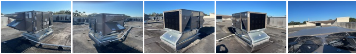
All 5 Sides of Installed Unit of RTU - Including Top with Condensor Fan Section.
