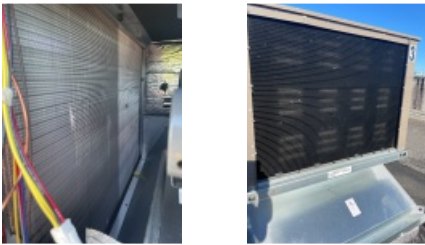
Complete / Clear Pictures of All RTU Condenser Coil and Evaporator Coil Surfaces.
