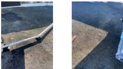
Roof Areas Around RTU Unit Showing the Areas are Clean and Free of Any Debris or Damage Related to the Installation.
