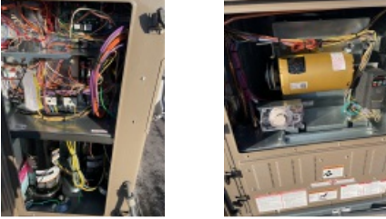
Interior Pictures of RTU Blower Section, Power / Control Section, Heat Section, Compressor Section.
