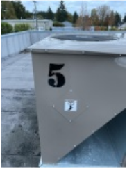
RTU Label Photo
