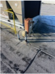
All RTU Electric and Heat Utility Piping Through Roof and All Connections / Penetrations at the Unit.
