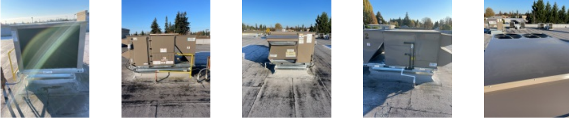
All 5 Sides of Installed Unit of RTU - Including Top with Condensor Fan Section.
