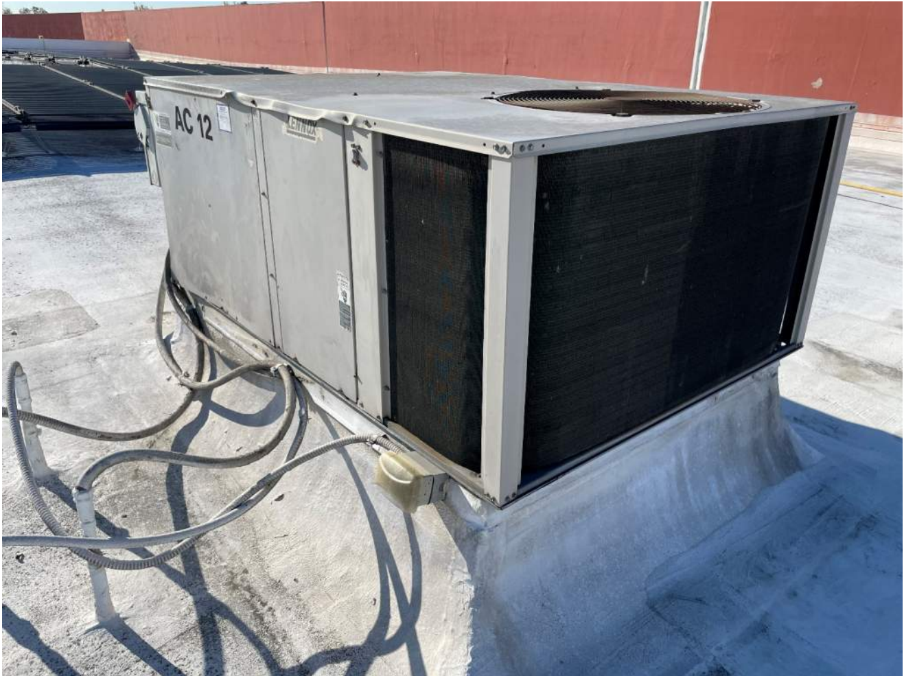
Photograph 9 – RTU #12. (RTU 13 Not Pictured)
