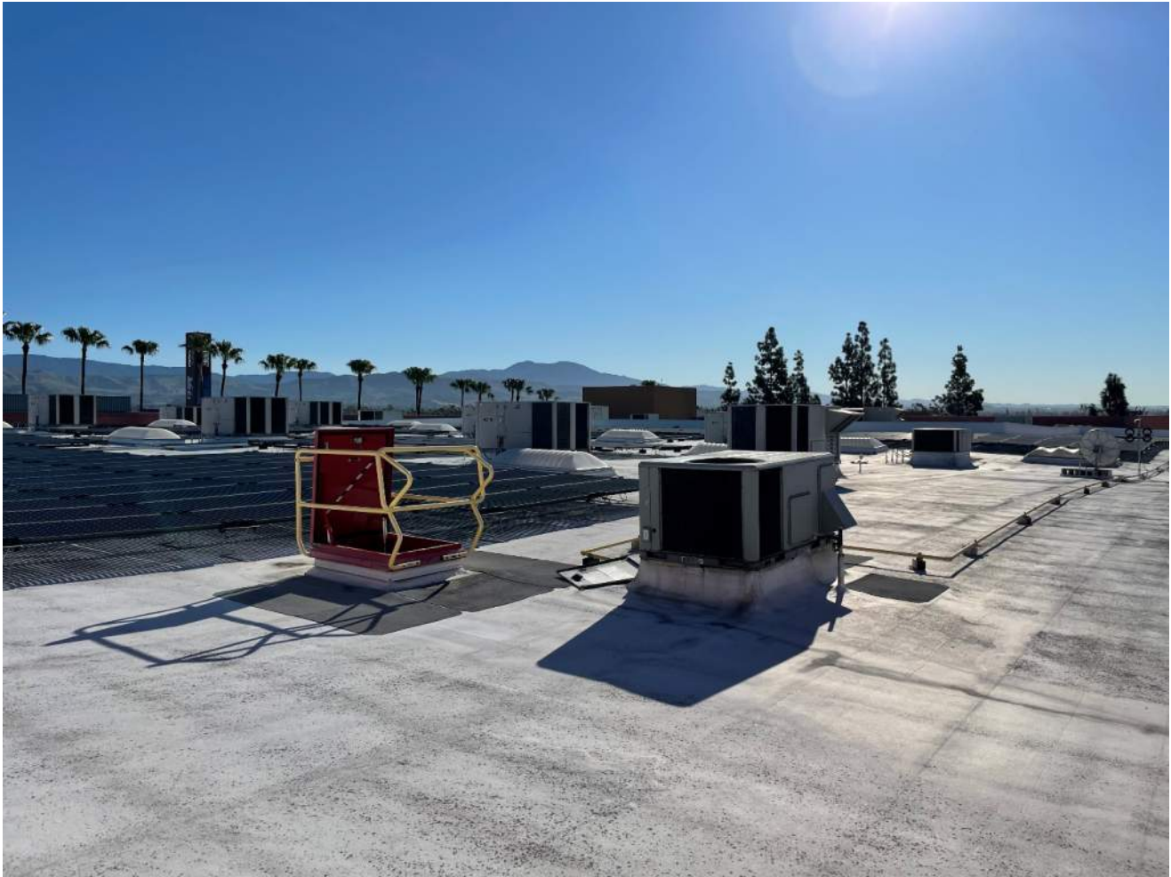
Photograph 6 – Overall view of units on roof. Screened in all directions by existing parapet walls
