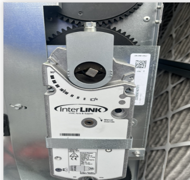
Actuator not secured 07/16/2023
