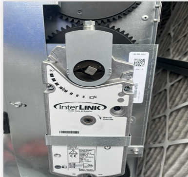
Actuator not secured 07/16/2023
