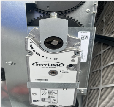
Actuator not secured 07/16/2023
