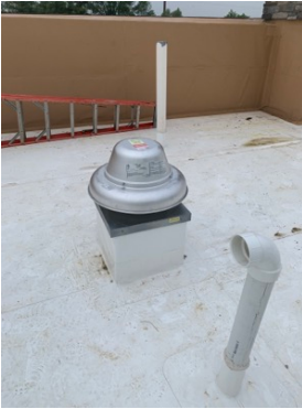
PRV-1 Serves restroom
