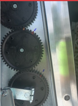
MARKED DAMPER POSITION
