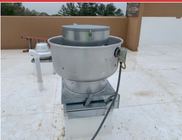
PRV-2 Serves Griddle hood
