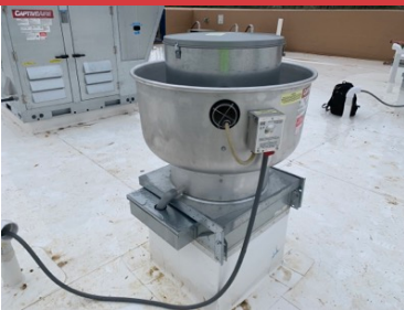
PRV-3 Serves Fryer hood
