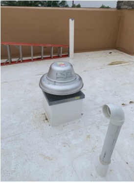
PRV-1 Serves restroom
