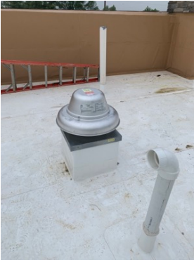
PRV-1 Serves restroom
