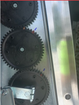
MARKED DAMPER POSITION
