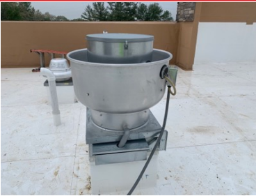
PRV-2 Serves Griddle hood
