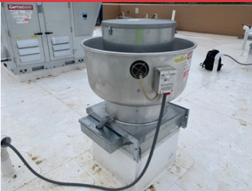
PRV-3 Serves Fryer hood
