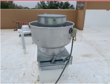
PRV-2 Serves Griddle hood
