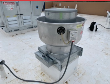
PRV-3 Serves Fryer hood
