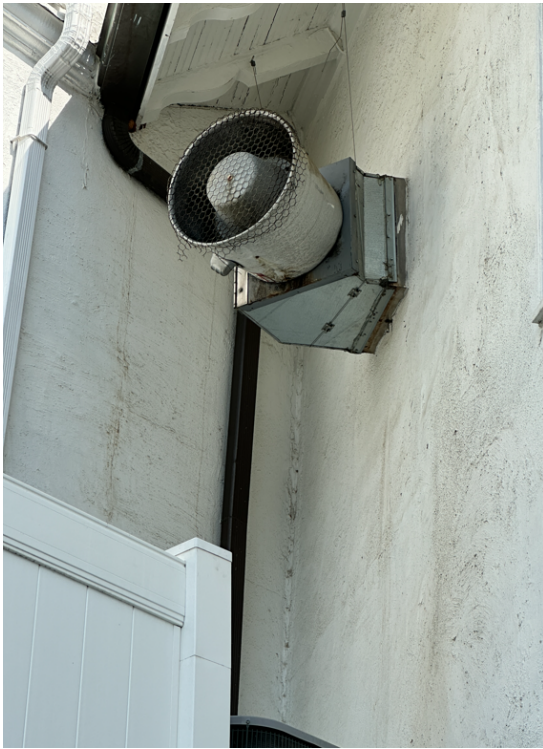
Dishwasher fan wall mounted up high on external wall.
