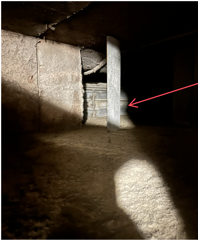
picture of inside the outside air duct looking inside - OA damper fully closed.
