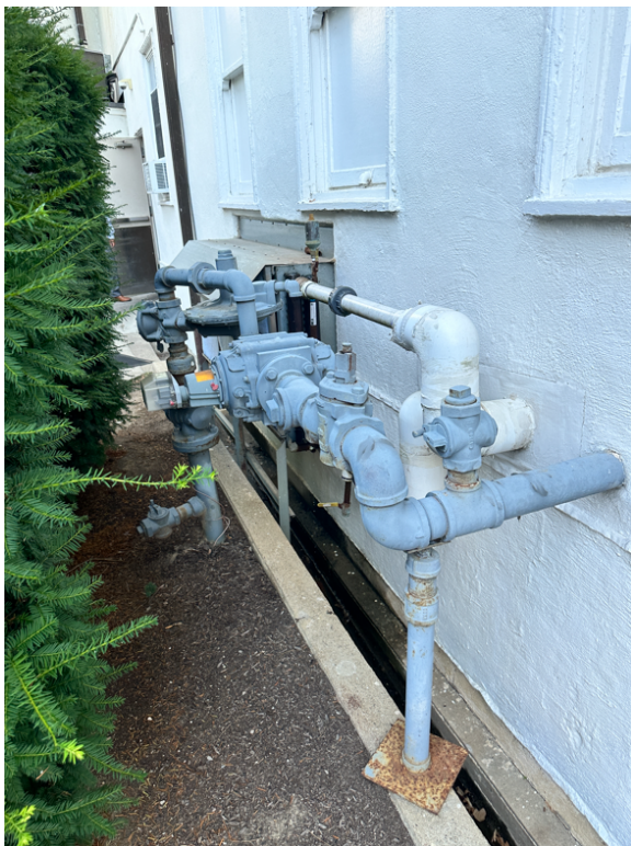
Main gas line just outside to the right of the OA Duct for kitchen.
