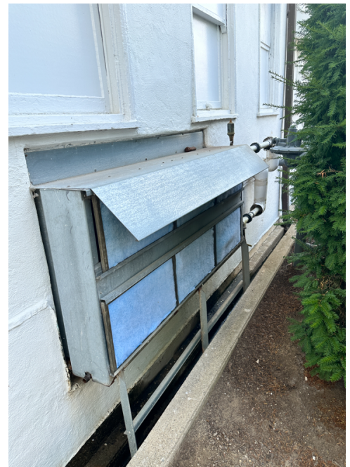
cooling coil mounted on inlet of supply duct of AHU for Kitchen.
