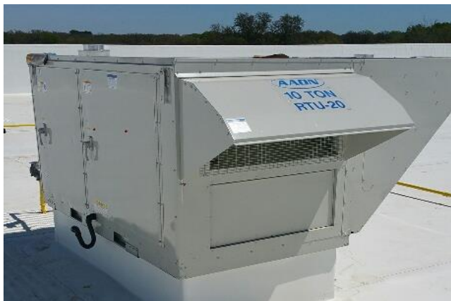
RTU 20 (TYPICAL 10-TON)
