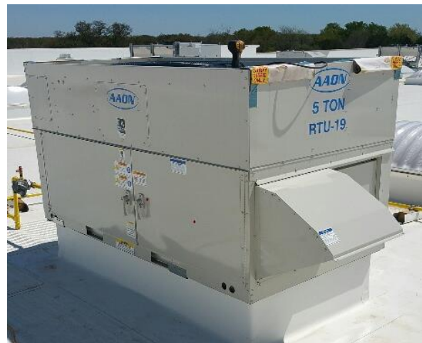
RTU 5 (TYPICAL 5-TON)
