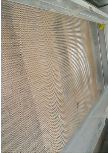
DIRTY DX COILS PHARMACY RTU
