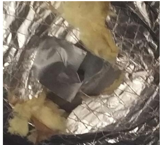
MEZZANINE BREAK RTU DIFFUSER 3 IS MISSING A DAMPER HANDLE. THIS IMAGE IS SHOWING THE DUCT TAPE THAT WAS PLACED ON DAMPER TO KEEP IT IN POSITION.
