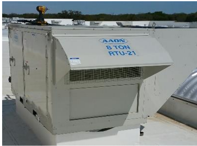
RTU 21 (TYPICAL 8-TON)
