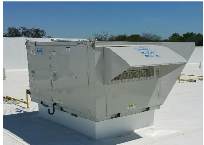
DELI RTU (TYPICAL 15-TON)
