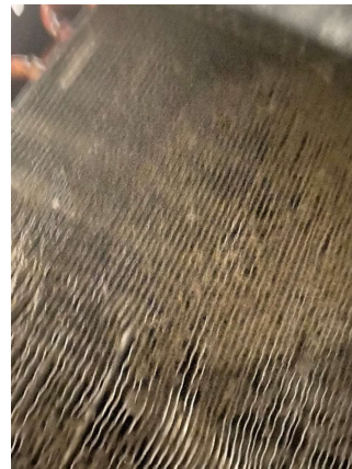
DXC-4 (MEAT COOLER 2) CLEAN CONDENSER
