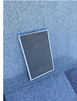
RTU-3 (DINING/RR) CLEAN OUTSIDE AIR FILTERS
