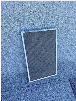
RTU-3 (DINING/RR) DIRTY OUTSIDE AIR FILTERS
