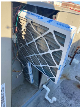
RTU-1 (DINING) DIRTY EVAPORATOR FILTERS
