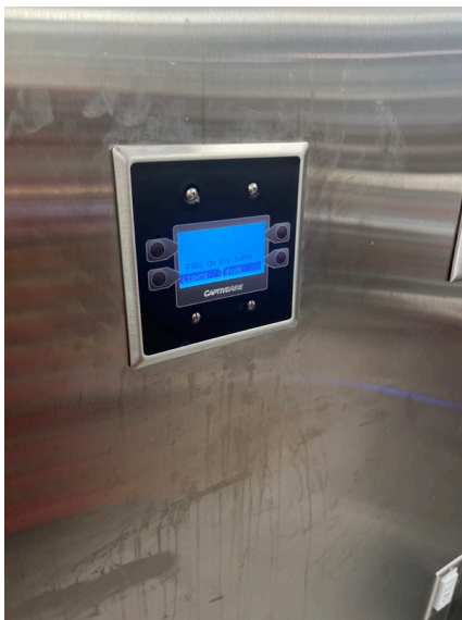
Captive Aire Hood HMI
