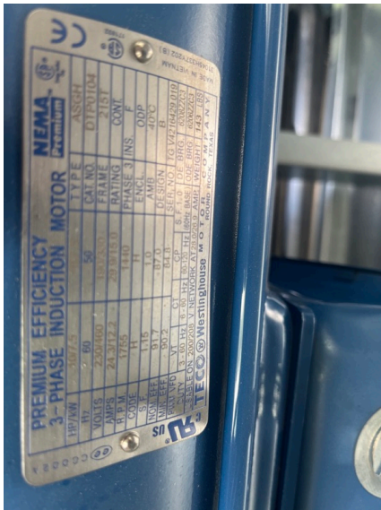
RTU-1 Motor nameplate
