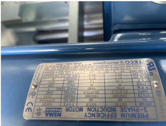
RTU-2 Motor nameplate
