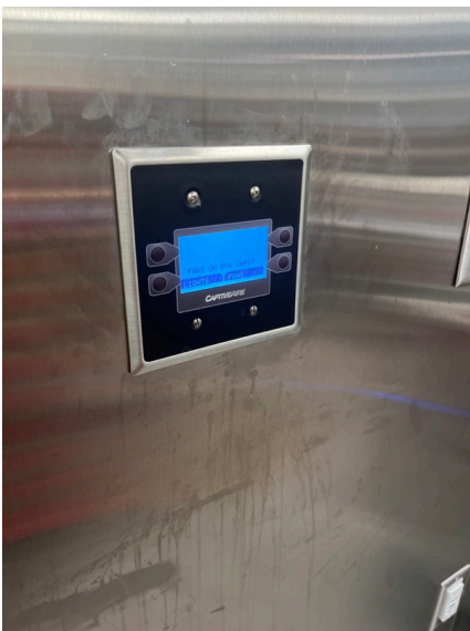
Captive Aire Hood HMI
