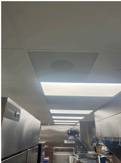
RTU-2 Cookline diffusers perforated.
