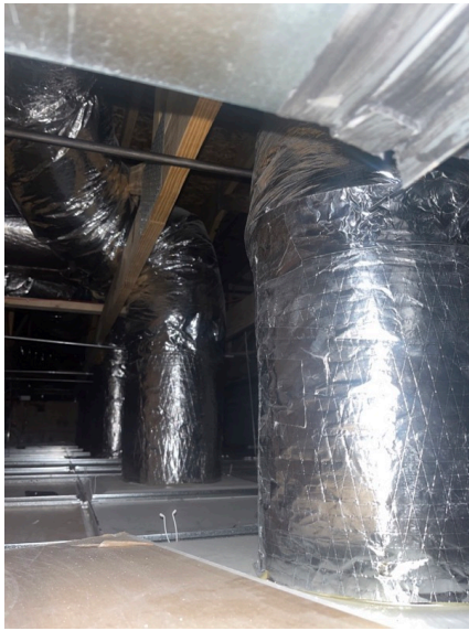
RTU-2 Cool line diffuser installation correct
