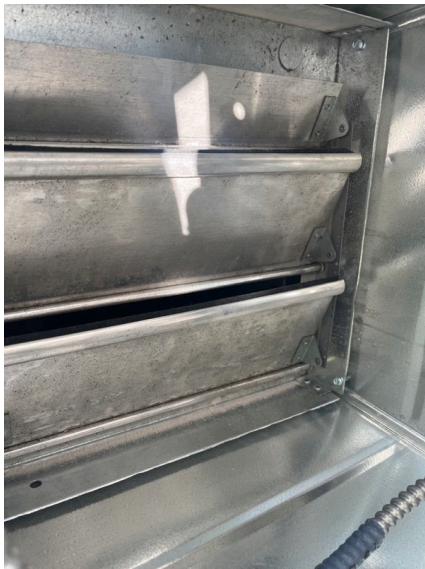
PRV-1 Backdraft damper installed and able To move freely.
